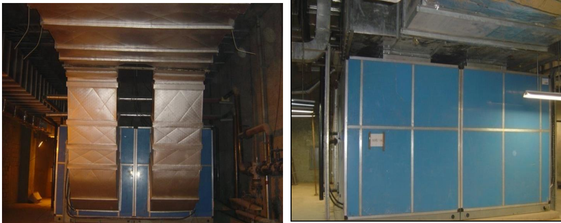
FIGURE 13.1: CONCOURSE AIR HANDLING UNIT
