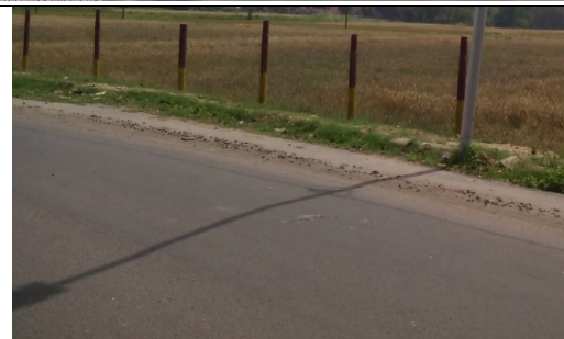
2. Absence of pedestrian facilities
