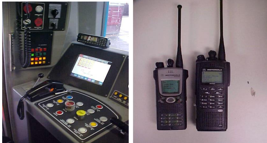
FIGURE 9.1: TRAIN CAB RADIO AND COMM. FACILITY FOR MAINTENANCE
