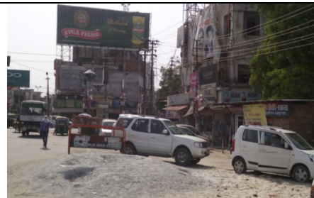
4. Encroachment of road shoulder
