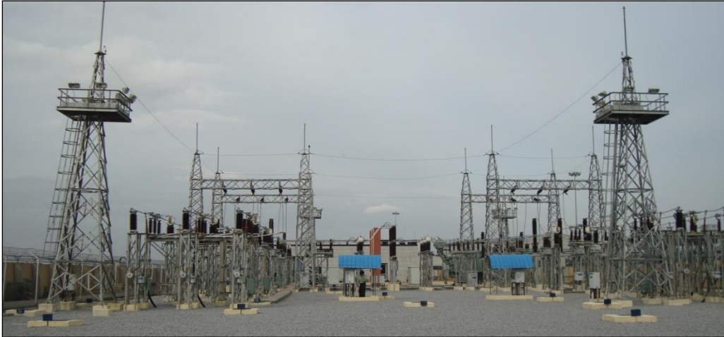
FIGURE 12.2: TYPICAL HIGH VOLTAGE RECEIVING SUB-STATION
