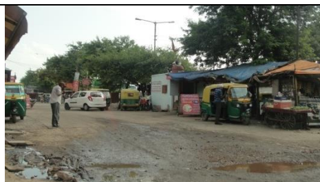
4. Damaged road surface leads to accidents.
