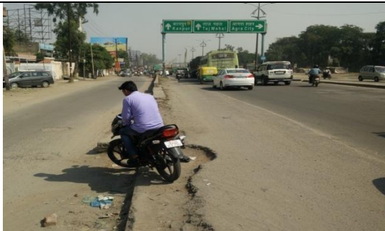
3. Damaged road infrastructure leads to disobedience of traffic rules by road users.
