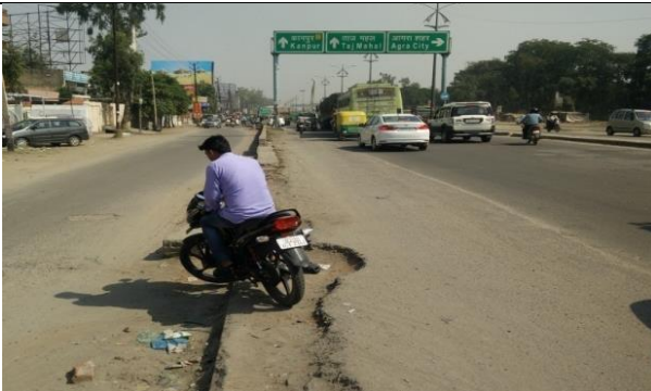
Shastri Nagar - damaged road infrastructure
