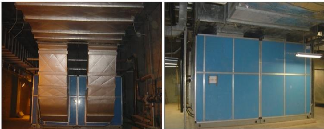
FIGURE 13.1: CONCOURSE AIR HANDLING UNIT
