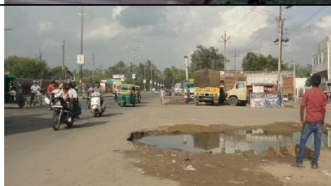
1. Damage road surface causes accidents
