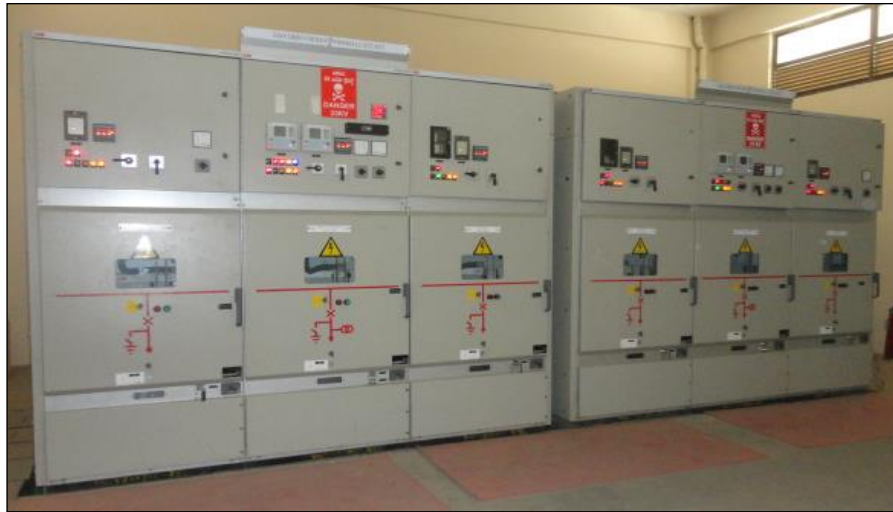
FIGURE 12.5: TYPICAL INDOOR AUXILIARY SUB-STATION
