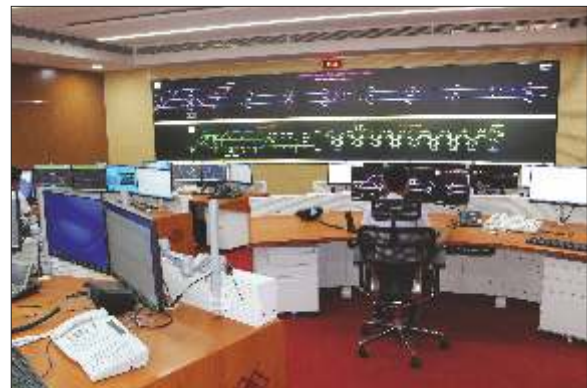
Signalling and train control system
