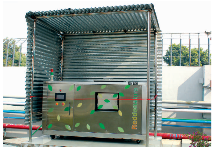
Automatic Waste Composting Machine at Depot
