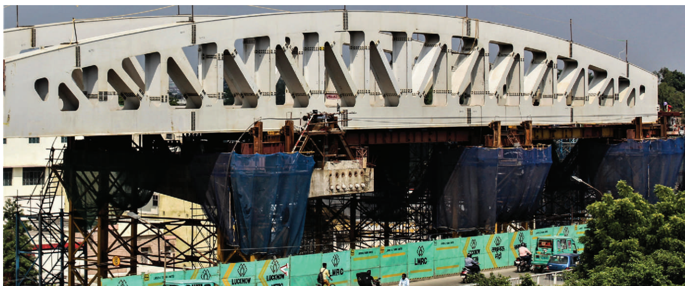
Erection of 60 Meter Special Steel Span near Nishatganj over the main line Railway operational track
