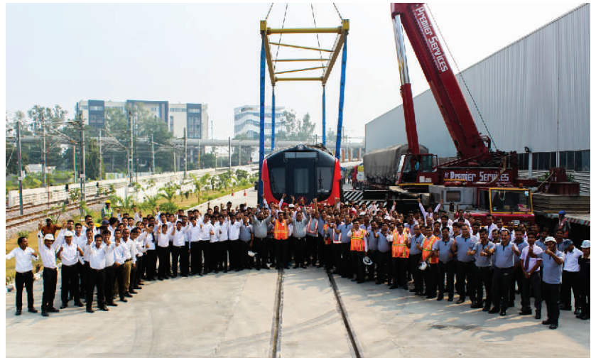
The LMRC Team with Managing Director, during the unloading of 20th Rolling Stock (Metro Train)
