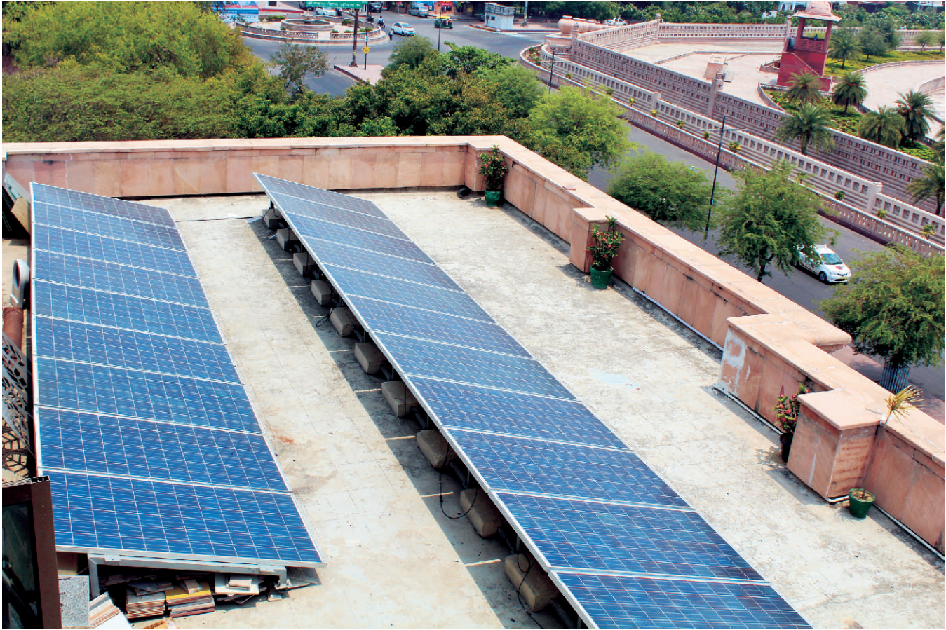
Solar panel at the Roof of Metro's Registered Office
