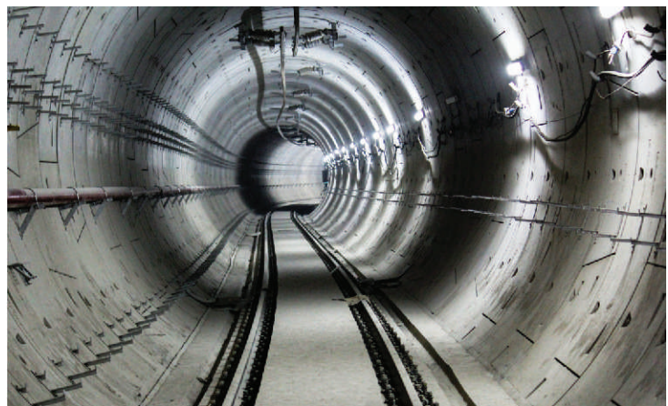
Work of Rigid Overhead Conductor System (ROCS) Inside Metro Tunnel Between Sachivalaya and Hazratganj.
